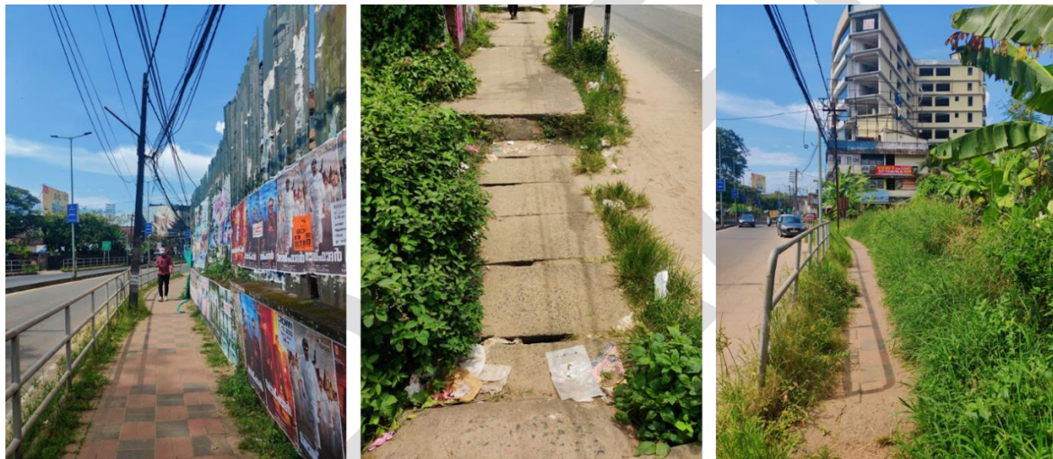
Figure 2-33 Condition of Footpath in Kozhikode City
