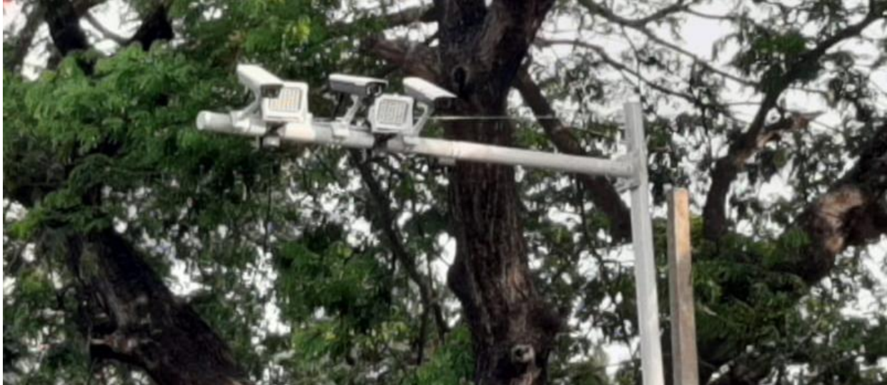
Figure 8-69 AI Cameras for Traffic Monitoring
