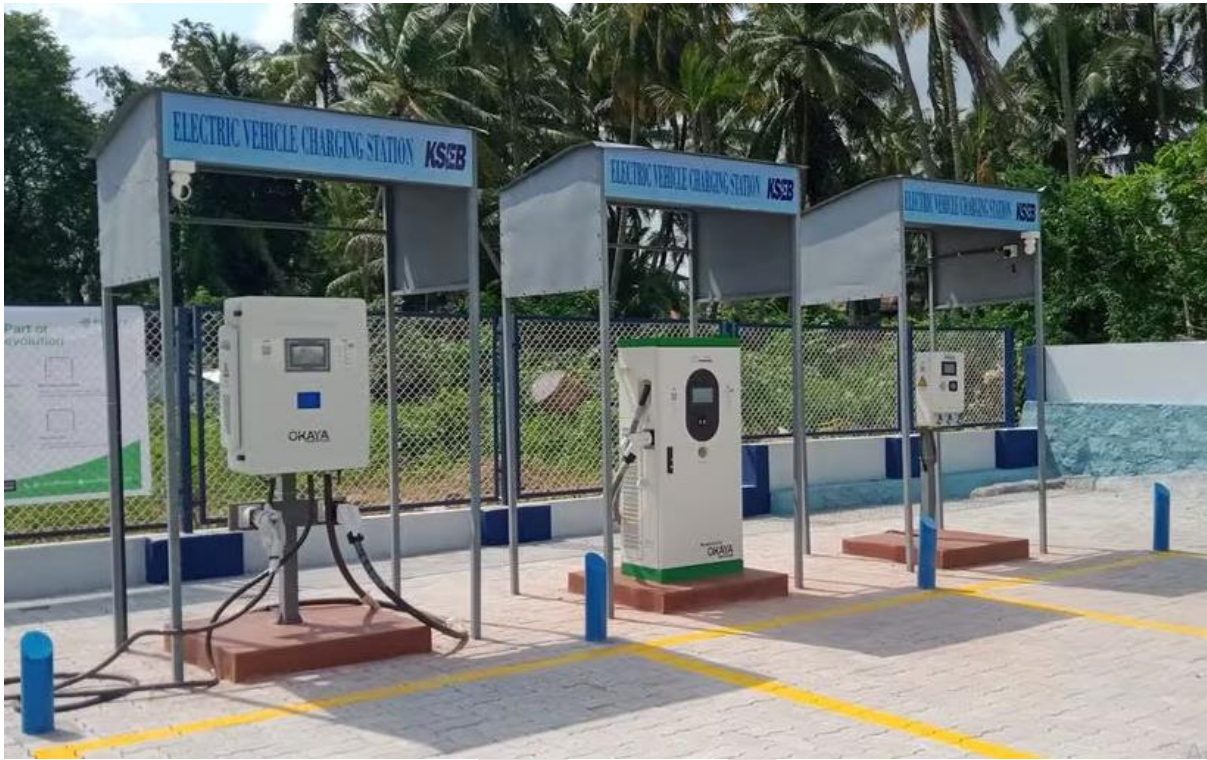
Figure 8-67 EV Charging Station at Kozhikode
